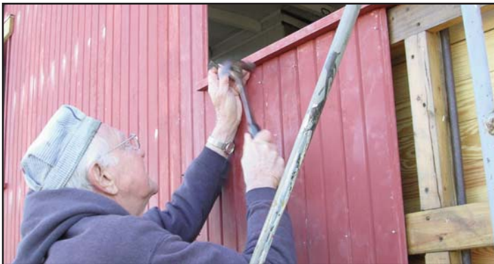
Gerry Herrmann, Project Manager, nailing siding on the NYC caboose. Photo courtesy of Bob Boothe.
