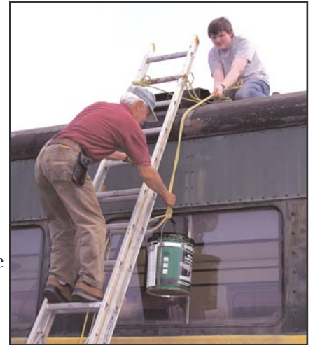
Dave Roberts and James Powell hoist a bucket of tar for applying to the roof of a passenger coach.
